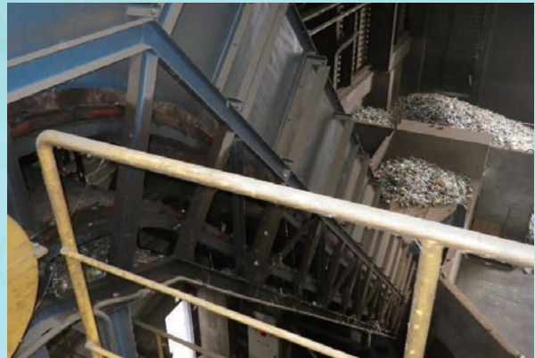
Crusher Feed Conveyor
