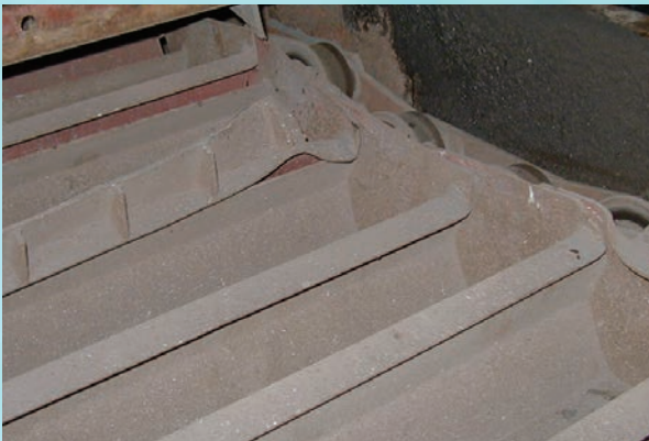
Non-burnable Trash Conveyor
